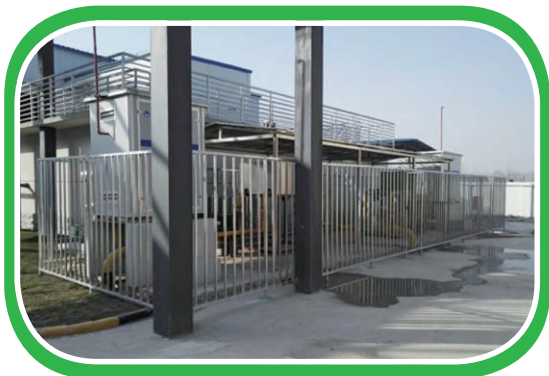
鍋爐燃氣調控站 Boiler gas control station
